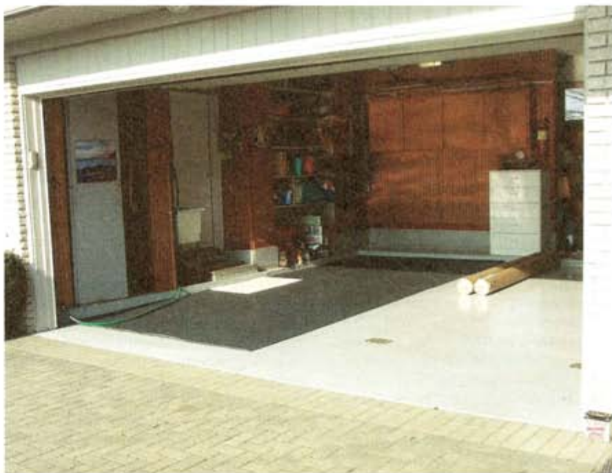
The new garage flooring was easy to unpack and install with the help of a second person.
